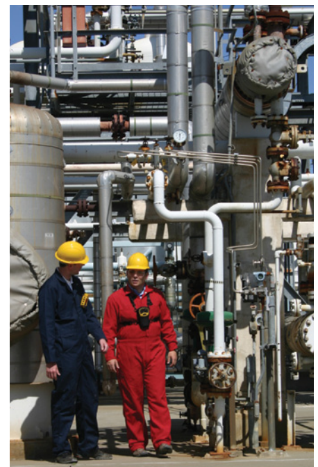
Fixed gas detection systems are used to protect personnel and equipment
